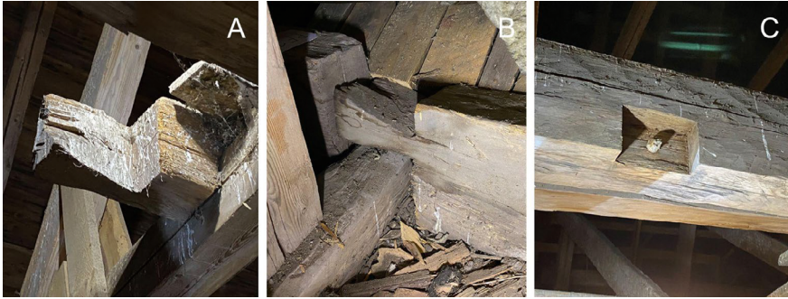
FIGURE 5 The reused timber in the nave roof structure of Pohja Church. (A) The joint of a wall log of the 14th century wooden church. The piece was reused as an anchor beam on the collar beams of the 1470s' structure © PANU SAVOLAINEN (2020). (B) The joint of a wall log of the 14th century wooden church. The piece was reused as an anchor beam on the wall plates © PANU SAVOLAINEN (2020). (C) A tie beam from the 14th century wooden church, reused as an anchor beam © PANU SAVOLAINEN (2020)
