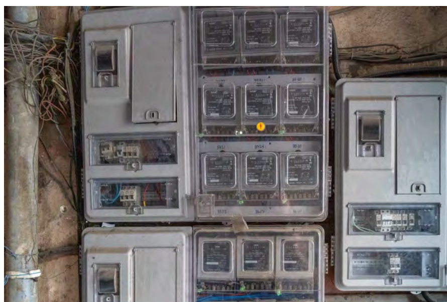
Residential electricity meters, Havana
