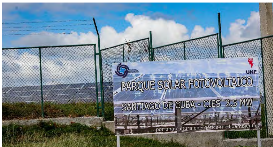
The solar power plant, Abel Santamaría
